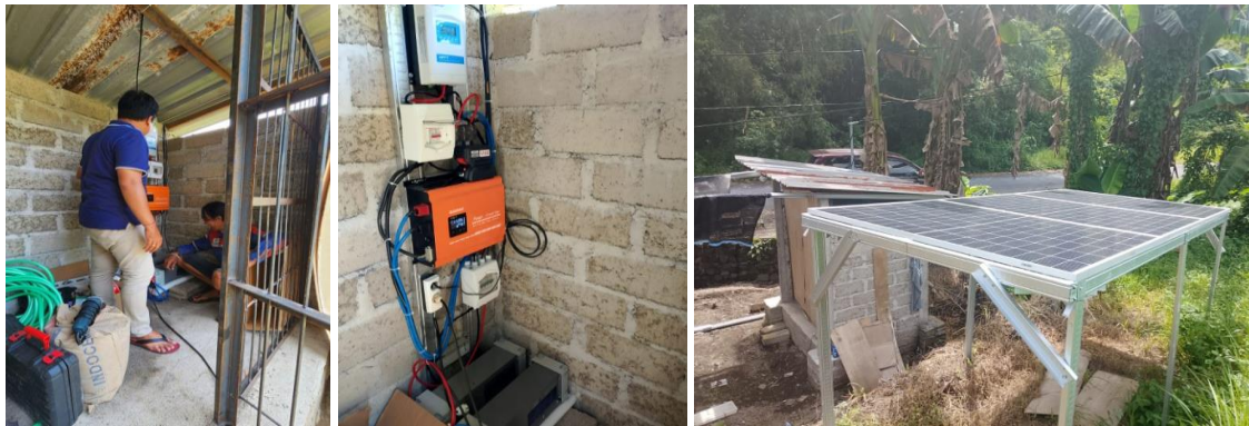
Gambar 4. Instalasi solar panel green energy
